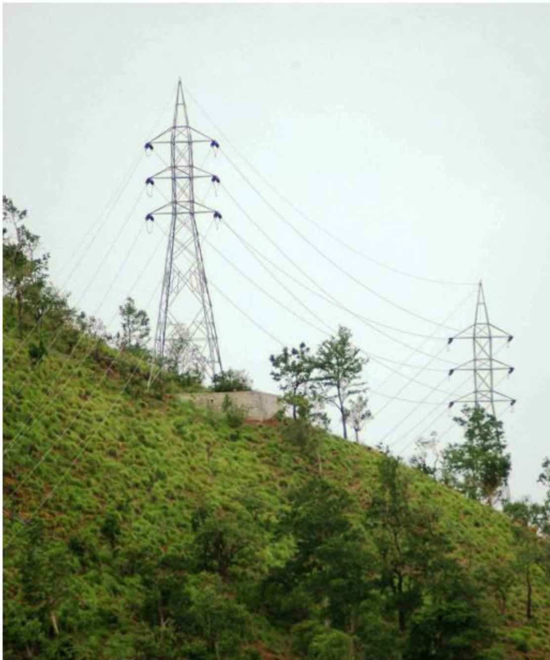
Figure 5-3: 132 kV line depicting actual position along with RoW and extent of damage
