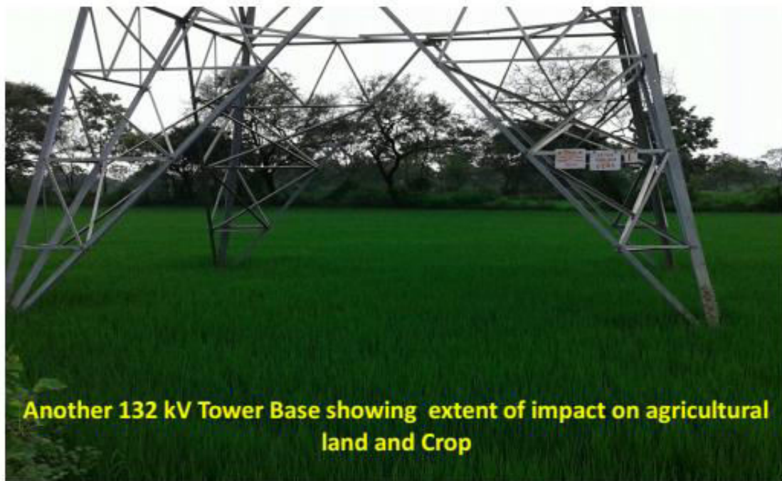
Figure 5-4: 132 kV Tower Base Showing Impact on Agricultural Land and Crop
