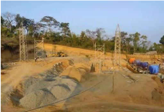
Switchyard of 132/33 kV Lungsen S/S
