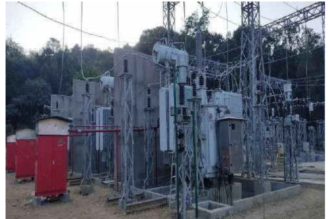
Switchyard of 132/33 kV Lunglei S/s
