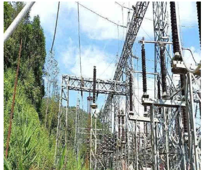
Switchyard of 132/33 kV Lunglei Extn. S/S
