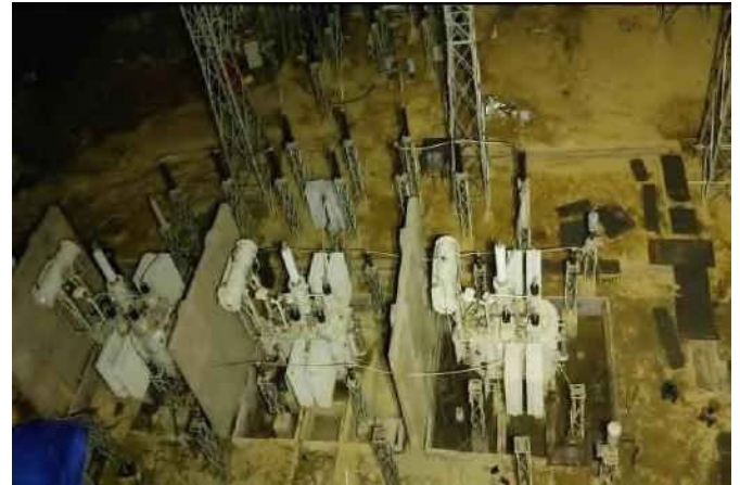
Switchyard of 132/33 kV Lunglei S/s
