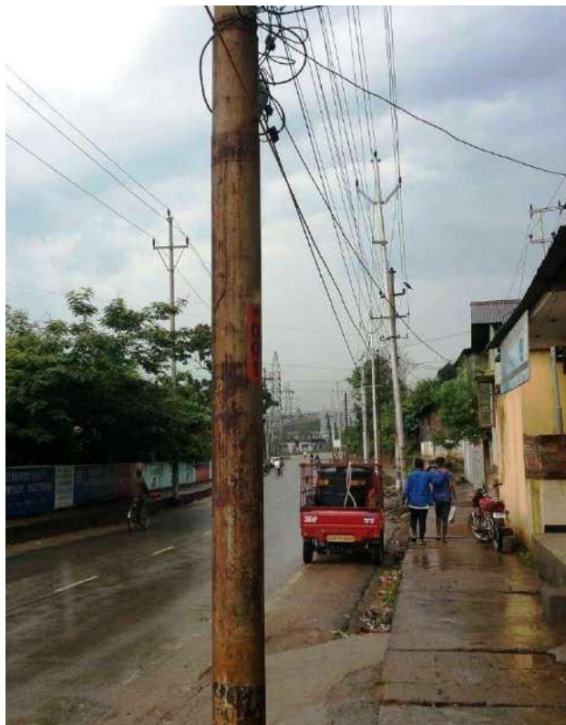
33kV line inside city area of Assam
