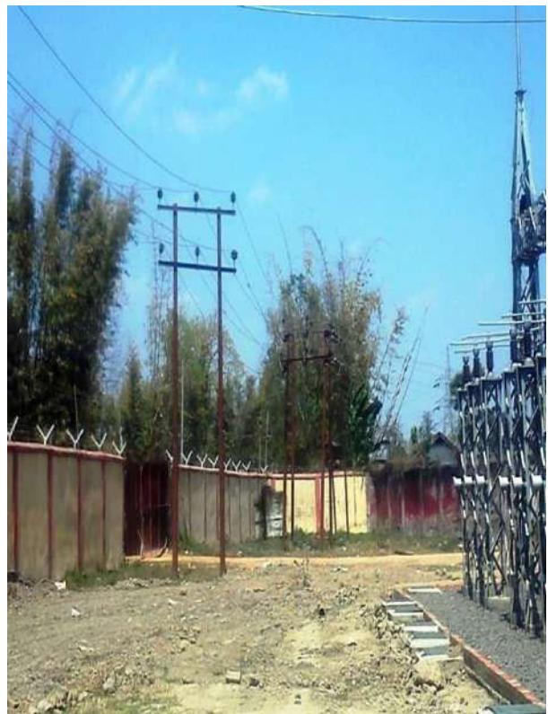
33kV (H Pole) line inside substation
