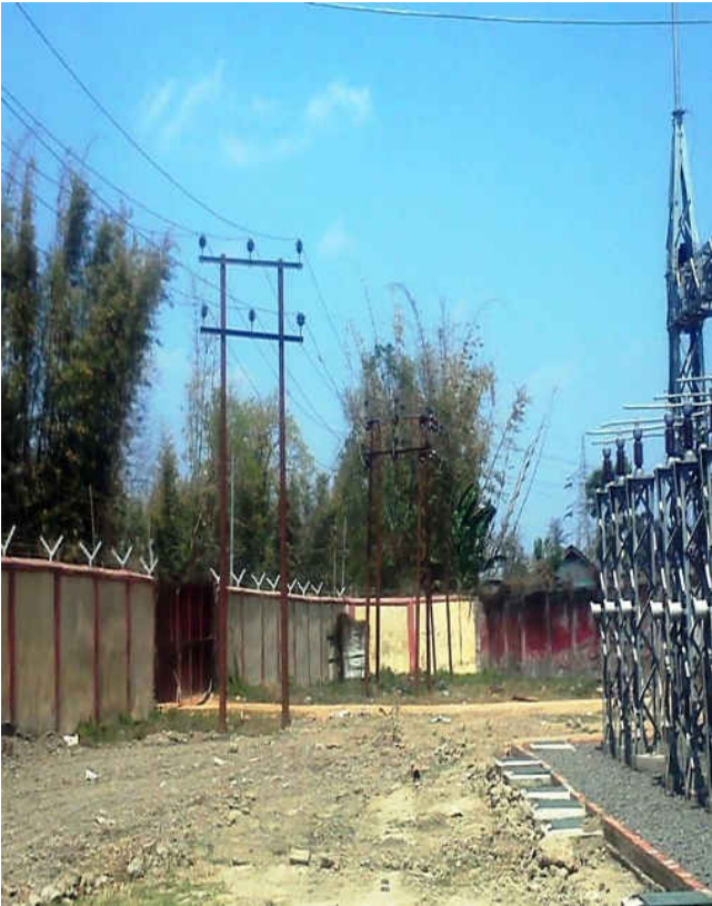
33 kV (H Pole) line inside substation
