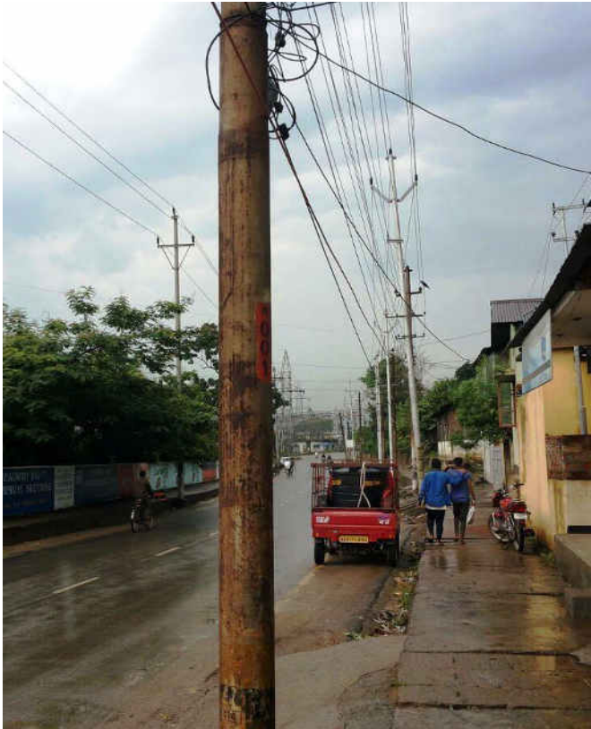
33 kV line inside city area of Assam
