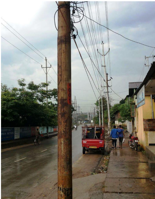
33kV line inside city area of Assam
