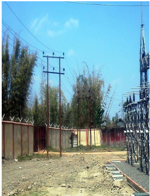
33kV (H Pole) line inside substation
